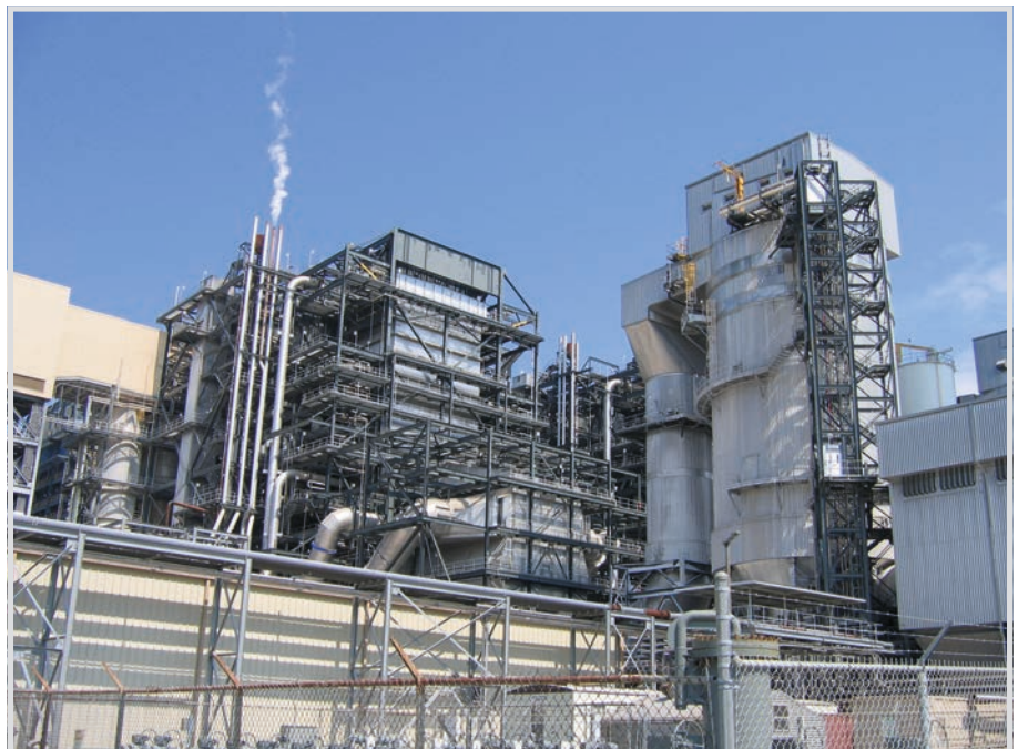
Fig. 6. World-class SDA. JEA's Northside Generating Station includes two Amec Foster Wheeler CFB boilers (2 x 300 MW units), each producing 831,000 ACFM of flue gas. Each boiler uses a single SDA followed by a pulse jet fabric filter to treat the flue gas produced by the pet coke- and coal-fired unit. SO 2 emissions are reduced up to 90 % and SO 3 , HCl, and HF emissions are reduced up to 99 %. Particulate emissions are 0.011 lb/MMBtu of fuel consumed. The SDA uses CFB fly ash only; no fresh lime addition is required. The plant has been in operation since 2002. Courtesy: Amec Foster Wheeler.
