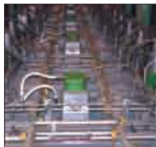
MasterCooler SMART® in Brammenanlage
